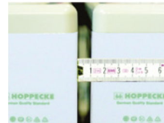
Fig. 5-14: 10 mm clearance between the batteries
